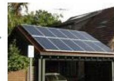
Solar Roof Top
